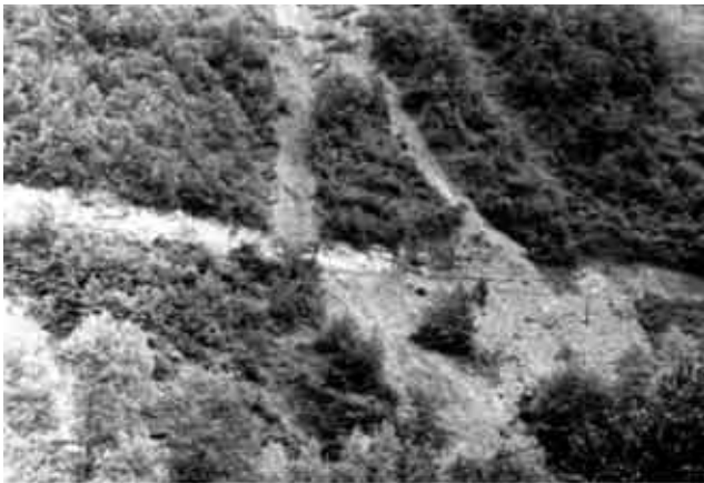
Figure 1 The slope damages during construction of forest roads
